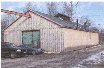
The old welding shop at Hahn & Schaffner was enclosed with board and batten siding in June 2010.
